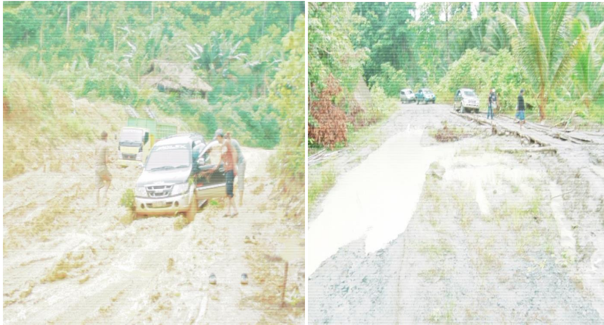
Road Conditions The Shaft Subaim (Halmahera Timur) – A (Halmahera Barat)
