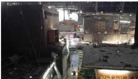
Figure 16. The deteriorating first floor and overlooking the random expansions done by tenants.
