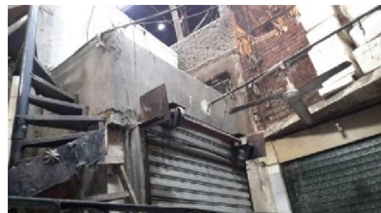
Figure 13. Unoccupied shops in the ground floor
