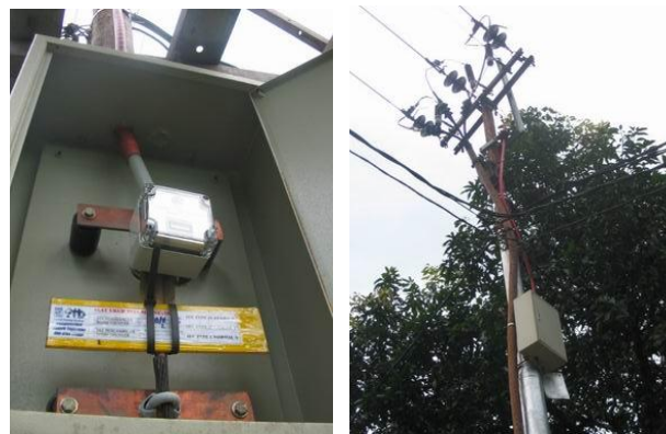
Figure 11 Magnetic tape measuring system and lightning event counter installation on arrester grounding lead.
