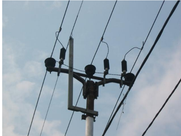
Figure 1 Typically overhead ground wire installation on the pole equipped with line arrester at Kapur feeder.
