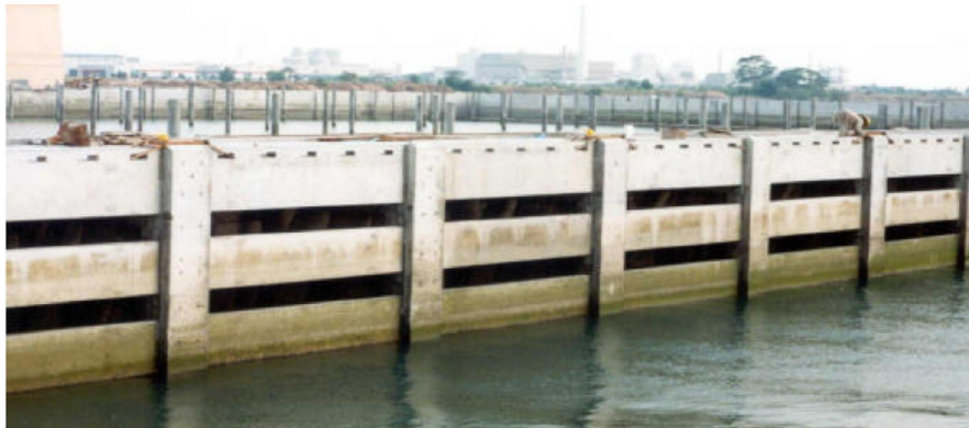
Figure 2 Example of the application of perforated breakwater (Raffles Marina Wharf/breakwater in Singapore).
