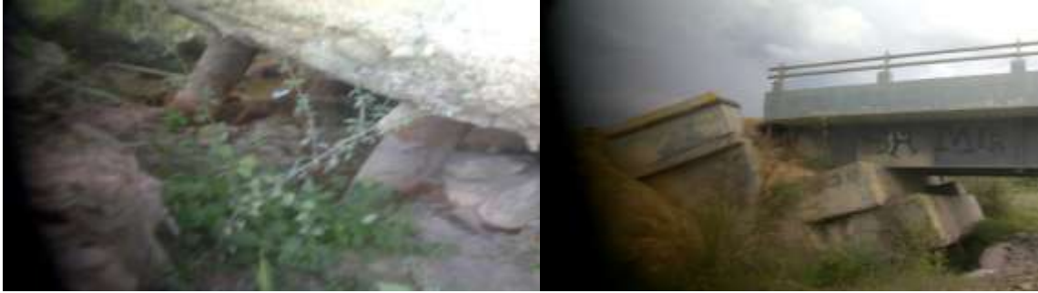
Gambar 1. Abutmen mengalami rotasi Gambar 2. Abutmen mengalami rotasi
