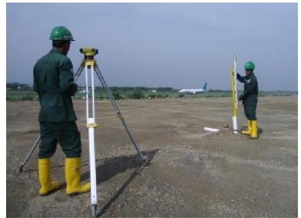
Gambar 42. Monitoring settlement plate
