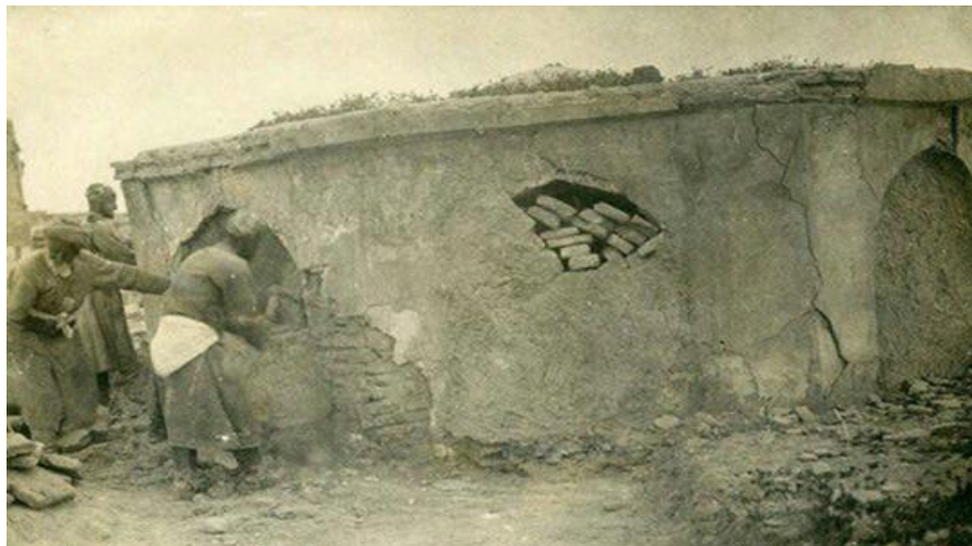
Restoration works at Magoki-Attari mosque. Dismantling repair plaster the beginning of work on. 1930s. 1934-1935
