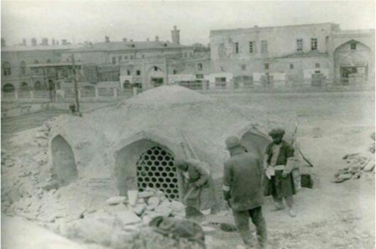
Restoration works at Magoki-Attari mosque. Dismantling repair plaster the beginning of work on making. 1930s. 1934-1935
