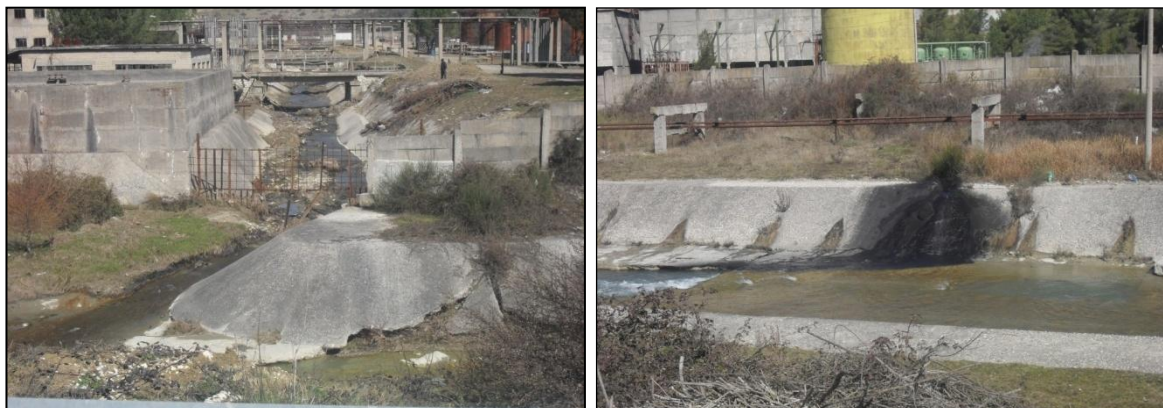
Figure 1: Direct discharged in Gjanica River of polluted water without passing through wastewater treatment plant of refinery, Ballsh.
