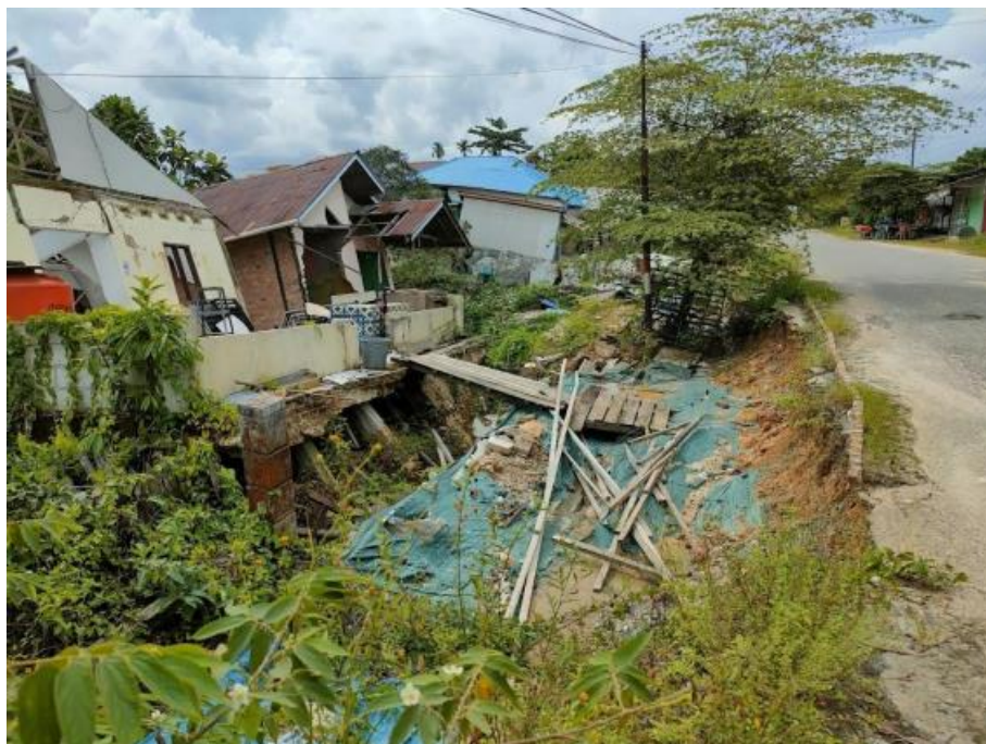
Gambar 1. Longsor di RT. 33 Jalan Sei-Wain Km.15
