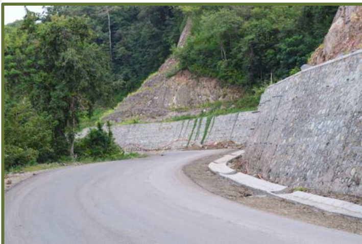
A PT Conbloc Infratecno road construction project in Flores. Courtesy of Alpino Iskandar.
