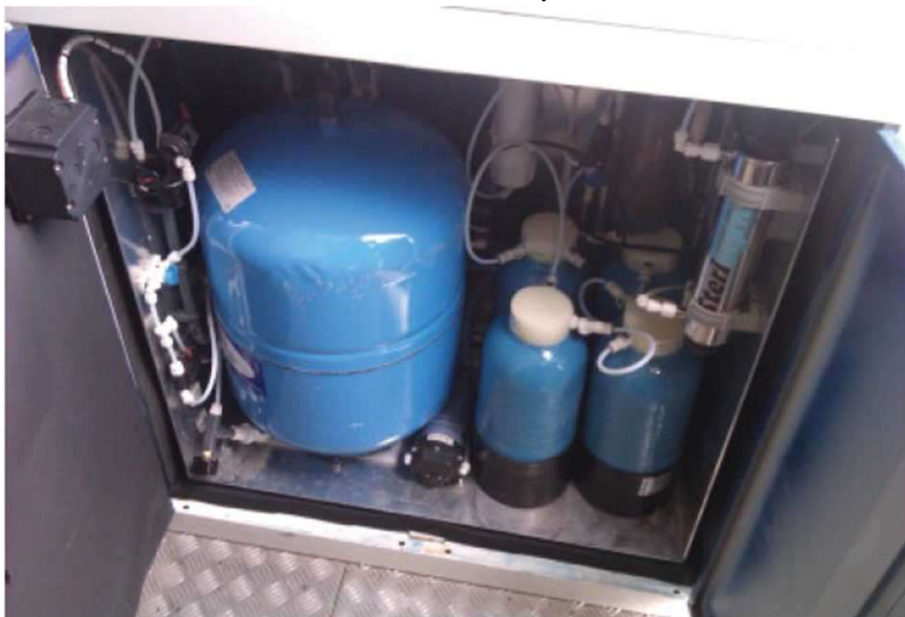
Picture 1. Water treatment. Courtesy of Dr. A. Cruden.
