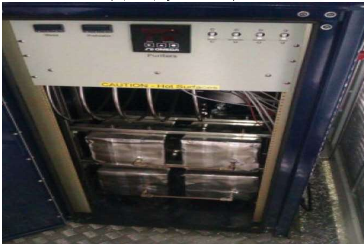
Picture 2. Dryer/heater/separator. Courtesy of Dr. A. Cruden.
