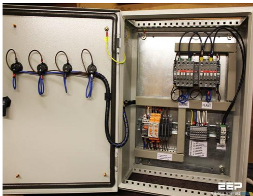
Gambar 1 Panel ATS (Sumber : electrical-engineering-portal.com)
