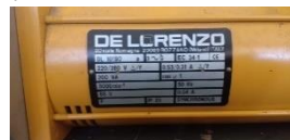
Gambar 4. Tampilan generator sinkron
