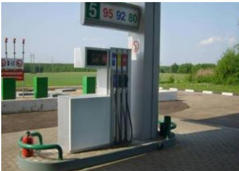
Figure 2: Island in YOSH and a fuel distribution column installed on it
