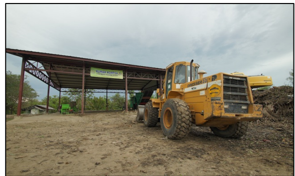
Figure 4. GJL wheel loader prepares soil and compost to cover the sanitary landfill (Faisal, 2014)
