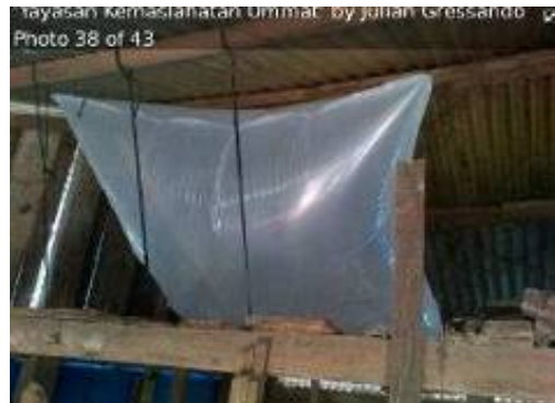
Fig 11 Reservoir with capacity 4000 l.
