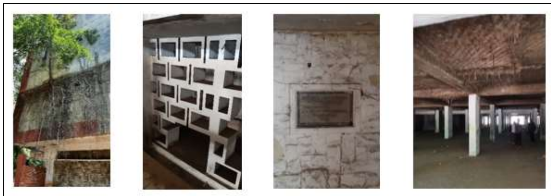
Figure 6. Living Tree on the Wall, Perforated Wall Motif, Building Inscriptions, Woven Bamboo Motif (Source: Survey result of the research team in 2020)
