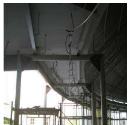
Figure 6. The steel portal beams are bent and dented
