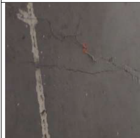
Figure 3. The occurrence of cracks in the span of the walls of shop houses (mostly due to tie beam structure)
