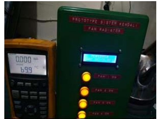
Picture 7. Fan Indicator Lights 4 Is On
