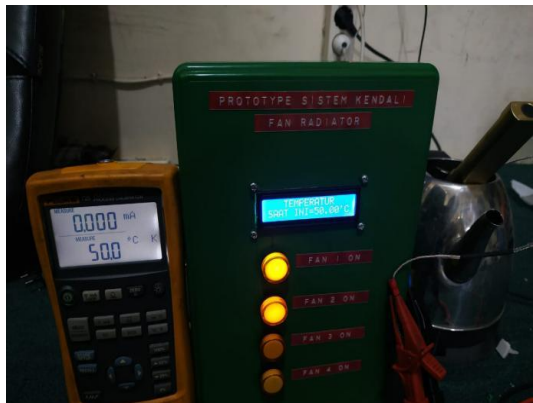
Picture 5. Fan Indicator Lights 2 Is On
