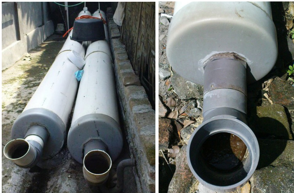
Figure 2. These PVC pipes are used by the community for the digester. They insert cow dung and water and the gasification processing will take from 1 to 2 weeks. Gadjah Mada University Indonesia's student fieldwork program (primarily students from the Livestock Department) introduced this gas plant. Japan International Cooperation Agency facilitated the initial installation by requiring only 30% of the project's capital investment from local people.
