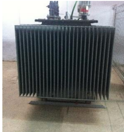
Gambar 1. Transformator 20/0.4 KV, 50 Hz, 800 KVA oil immersed,
