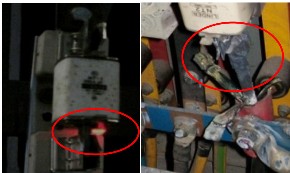
Gambar 2. Fuse Base Rusak
