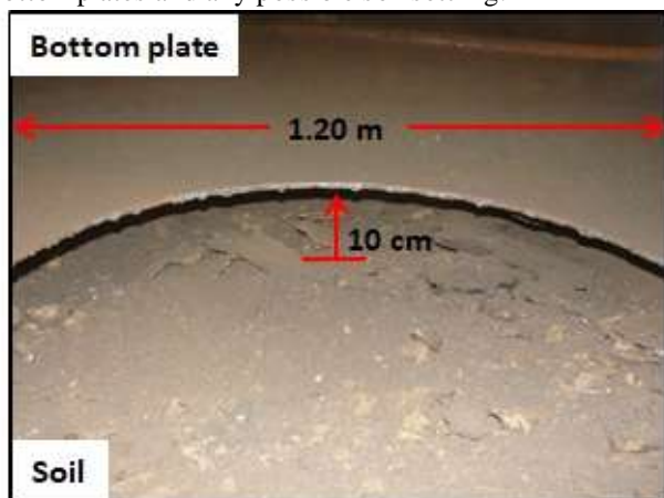
Fig.3: The void or gap between the bottom plate and the soil.
