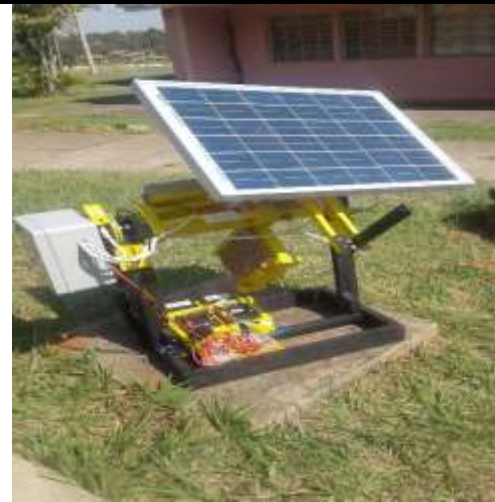
Fig. 1: Operational Automated Solar Tracker.
