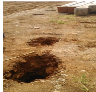
Gambar 10. Lubang akibat proses dolly
