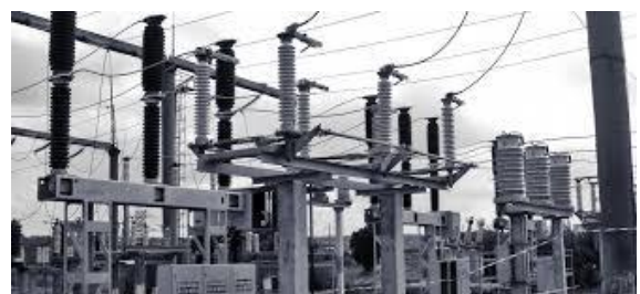
Fig. 1. A typical 132/20 kV high voltage substation (outdoor switchyard).
