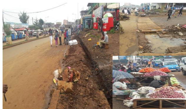
Fig. 3.1: Sidewalk quality problem, absence of buffer and presence of illegal occupancy on walkway in Nekemte city
