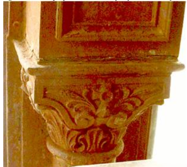
Figure 13: Example of the corrosion from the interior of the church, 2010
