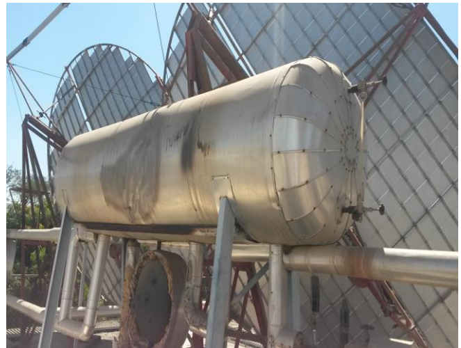
Fig.5 Water Storage device
