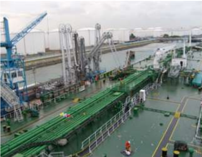
Gambar 3. Pipe line Inert Gas System di dek Kapal
