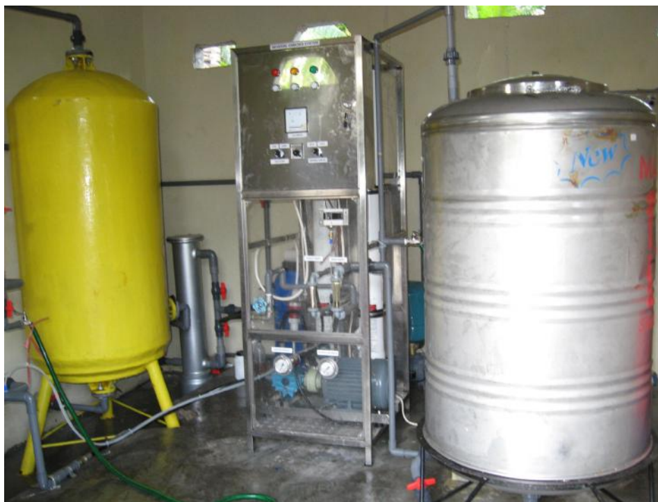
Gambar 18 : Unit Treatment Reverse Osmosis .
