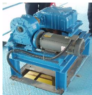
Mixer clarifier (MXC)
