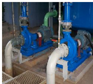
Pompa backwash filter (PBW)
