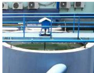
Mixer flocculator (MXF)
