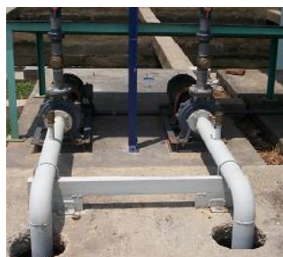
Pompa booster chlorine (PBC)
