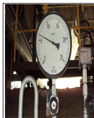
Gambar 3. Manometer Boiler Alstrom
