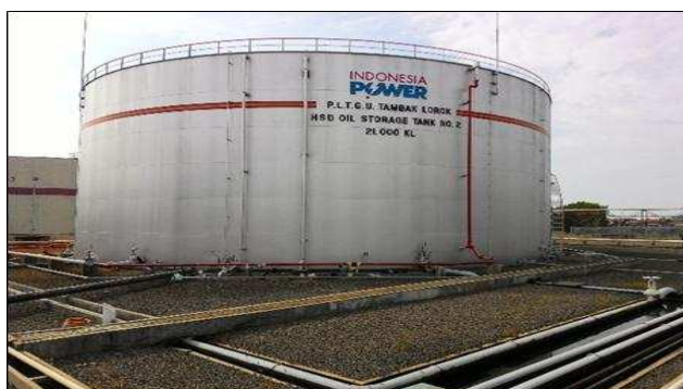
Gambar 1. HSD Oil Storage Tank
