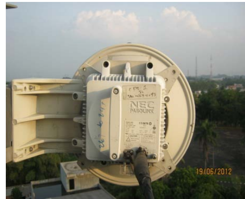
Gambar 4.7 Gambar instalasi Outdoor site JKT_06B1052 IBS BSD Junction
