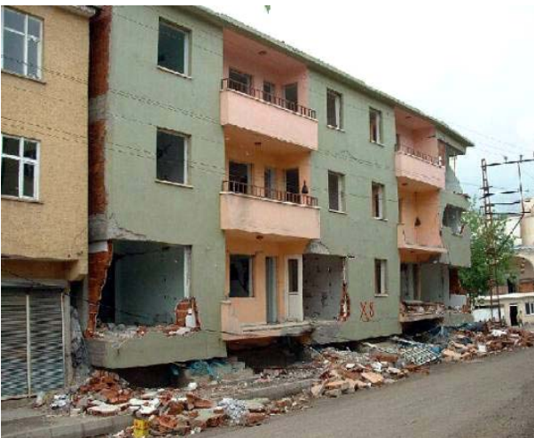
Gambar 1. Soft-storey - Gempa Bingol, Turki 2003
